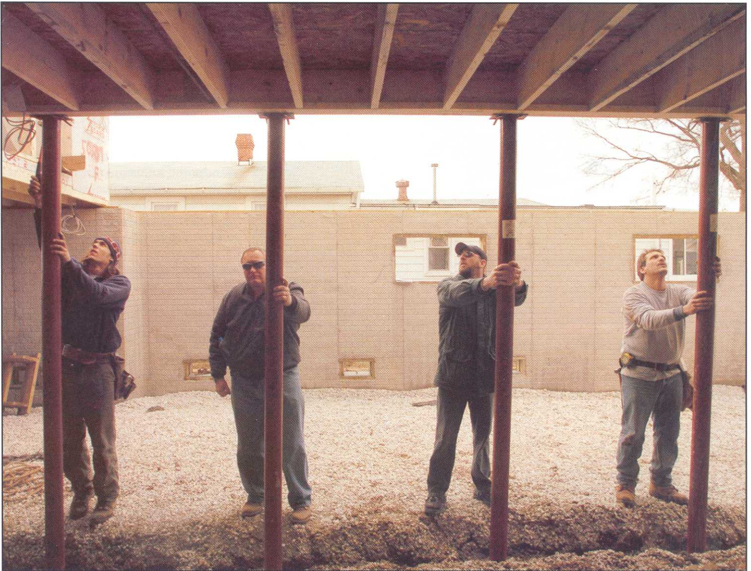
A crew positions a module on supporting columns while standing in basement of Middle River house. The home's modules included a high-end kitchen and a master closet as large as some bedrooms.
