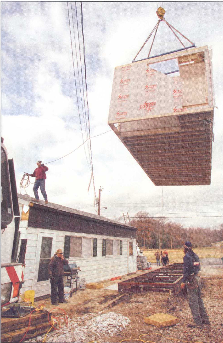
A crane lifts a modular section over power lines as a crew assembles a waterfront home in Middle River at the end of January. The 3,500-square-foot home was raw lumber the previous week.
